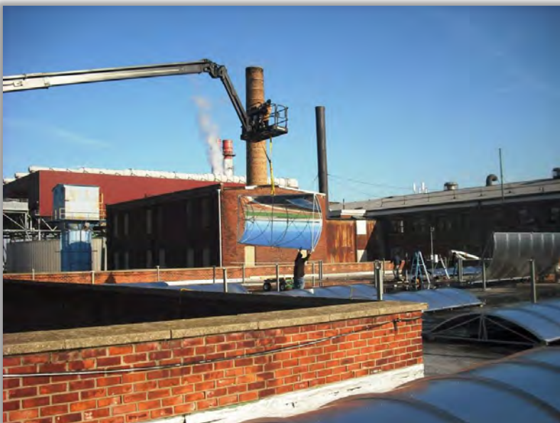
Workers install a solar cooling system on the Steinway & Sons piano factory in New York. (Steinway & Sons)
